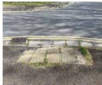
Misaligned tactile paving at the existing informal pedestrian crossing point to be corrected.
